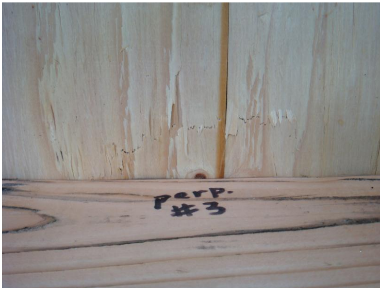
Figure 4. Buckled Plywood Shear Perpendicular to Rafter
