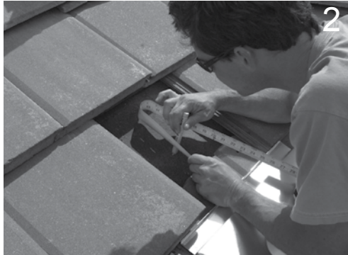
2 Remove tile at location of mount. Measure up 6 5/8" to center of mount. Measure 5 1/2" from exposed edge of adjoining right tile to center of mount, and mark paper. At this point you should install rafter blocks below all mount locations (See blocking instructions on page 2).
